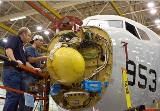
A Boeing and a Raytheon employee complete installation of an APY-10 radar antenna on P-8A Poseidon test aircraft T2
